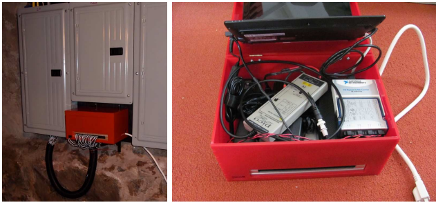
Figure 5: The REDDBox, installed in a home (left) and showing internals (right).
